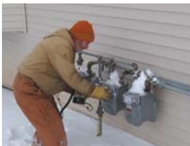
Rock Energy Cooperative employees completing the installation of Badger® ORION® modules on gas meters
