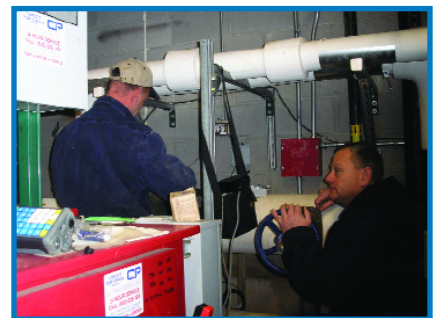
Dan Mann (right), Water Superintendent and Ron Alford, both of South Elgin Public Works, install a Badger® GALAXY® remote transmitter to a Recordall® Compound Series meter inside the high school.
