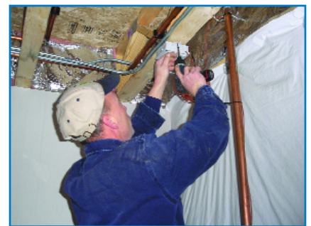
Ron Alford installs a remote transmitter in the floor joists of a newly constructed condominium.
