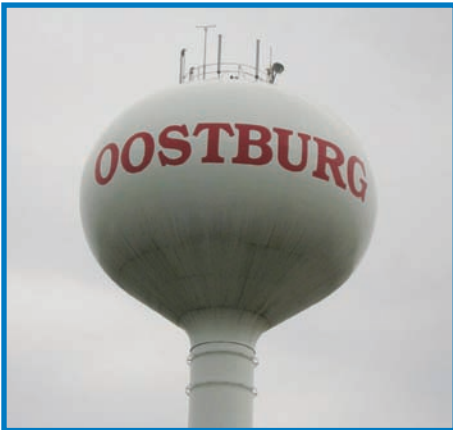
Badger ® GALAXY ® antenna mounted to the top of the Oostburg, Wisconsin water tower.
